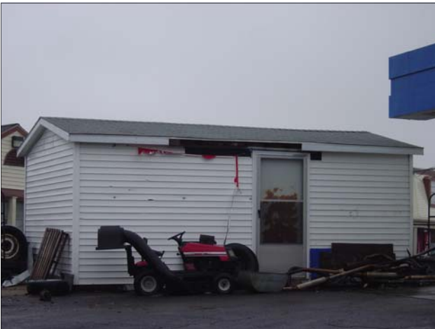
Damaged fascia and siding on storage building at Marathon Service Station lot. Note the outside storage of junk.
