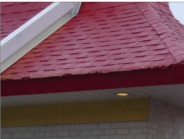
Deteriorated roofing material on McDonald's on east side of South Route 45.
