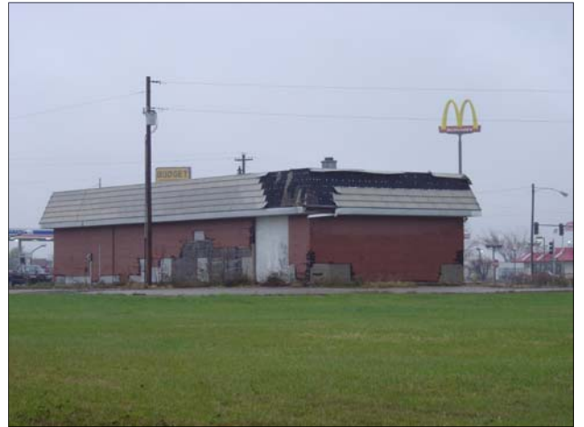
Deteriorated vacant service station at the southwest corner of Paradise Road and South Route 45.
