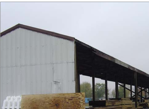
Damaged siding and fascia on lumberyard building.
