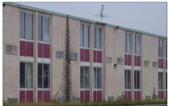
Rear of vacant hotel. Note water damage on bricks and mortar.
