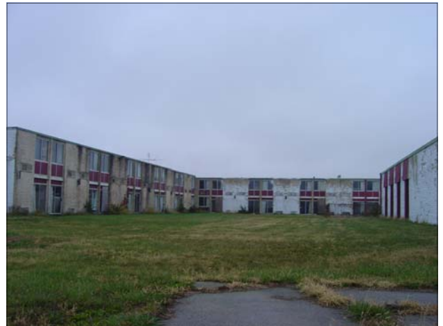
Peeling paint and deteriorated site of vacant hotel.
