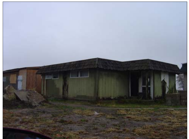
Dilapidated two-family apartment building on Carter Lane. Note deteriorated siding and broken windows.
