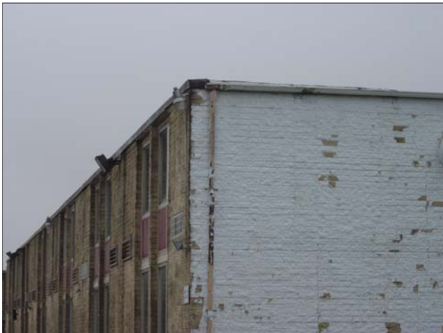
Peeling paint and deteriorated bricks and mortar on side of vacant hotel.
