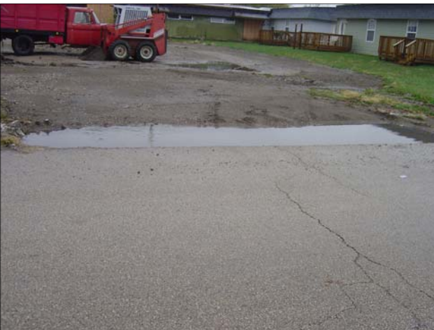
Deteriorated shoulder and insufficient drainage on Carter Lane.
