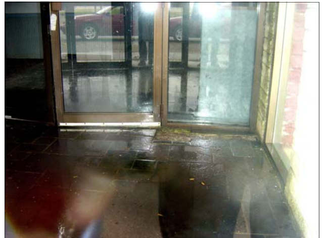
Standing water and broken floor tiles in entrance to vacant hotel.
