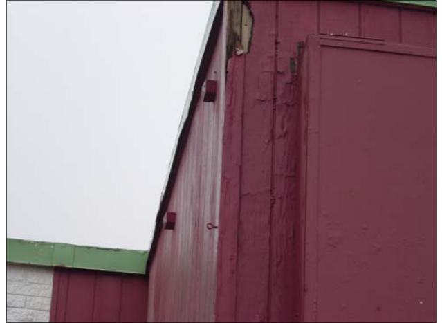
Peeling paint and deteriorated siding on front of vacant hotel.
