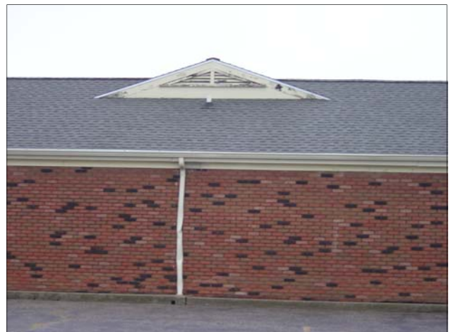
Peeling paint and damaged downspouts on apartment building.
