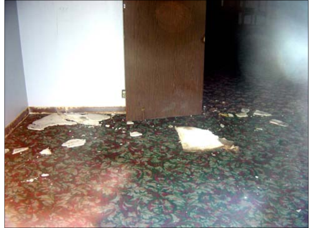
Falling ceiling tiles on floor of hallway in vacant hotel. Note the mold on the base of the walls.
