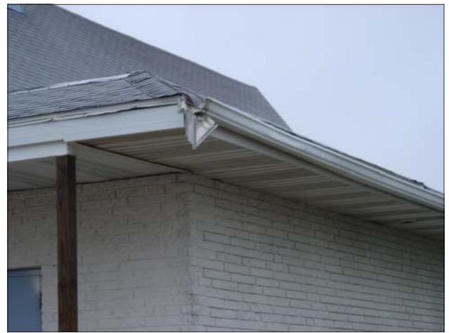
Damaged gutter on Budget Inn building.
