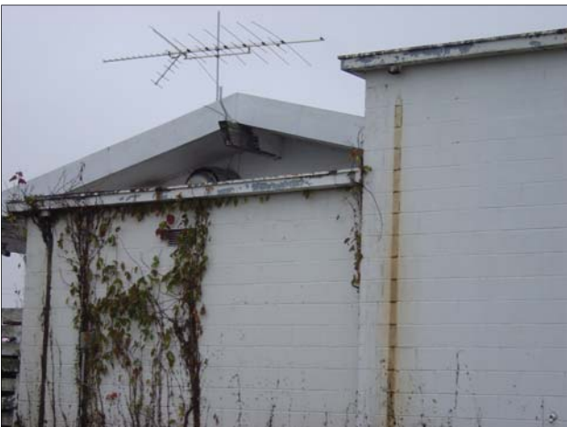
Rear of Marathon Service Station. Note the missing downspouts and deteriorated fascia.
